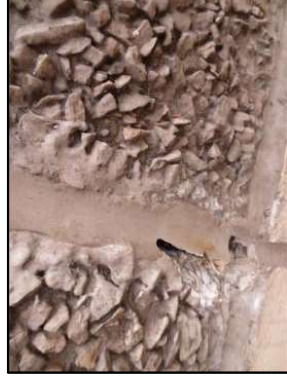
Photo N° 3193 ECH-N°15 -BAT 32-210 pignons Murs Joint de dilatation
