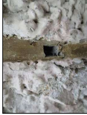
Photo N° 3189 ECH-N°12 -BAT 32-210 pignons Murs Joint de dilatation
